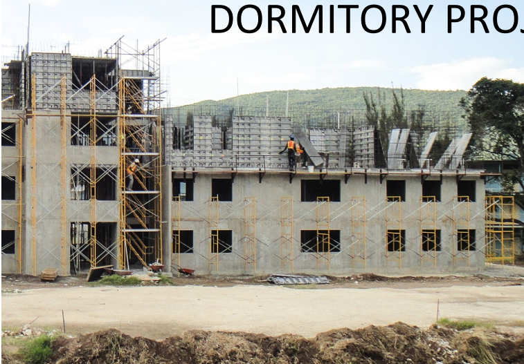
Progress after 5 weeks - 3 rd floor Forms not required to complete 3 rd floor were moved up to start the 4 th floor.
